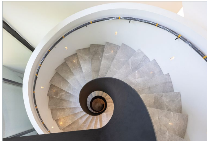
The sculptural spiral staircase of concrete that was cast onsite and features a balustrade crafted from a single curved metal sheet
